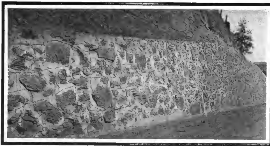
Excellent example of modern practice in making retaining walls to protect road surfaces
